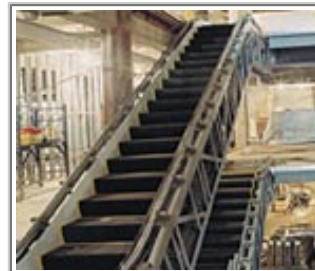
New escalator banks for improved vertical mobility.
